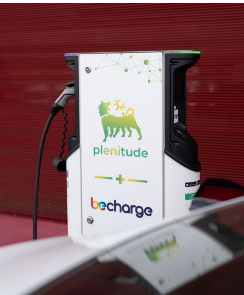
Be Charge charging point
